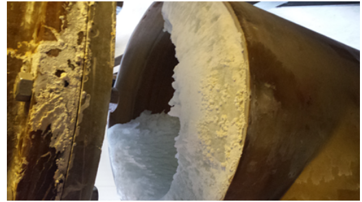
Fig. 4. Crystallizing salts in the pipeline
